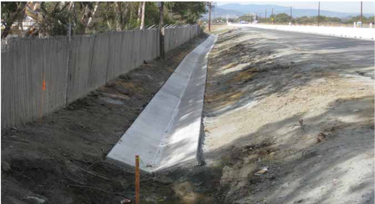
Minor Concrete at Tri Cal Lined V Ditch
